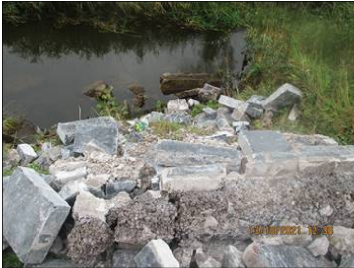
Plate 1.2 . Skeagh Bridge. Debris has fallen on embankment and instream resulting from fallen masonry parapet wall.
