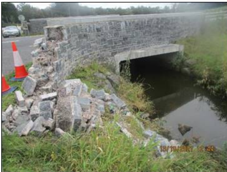
Plate 1.1 . Skeagh Bridge. Damaged parapet wall and fallen debris.
